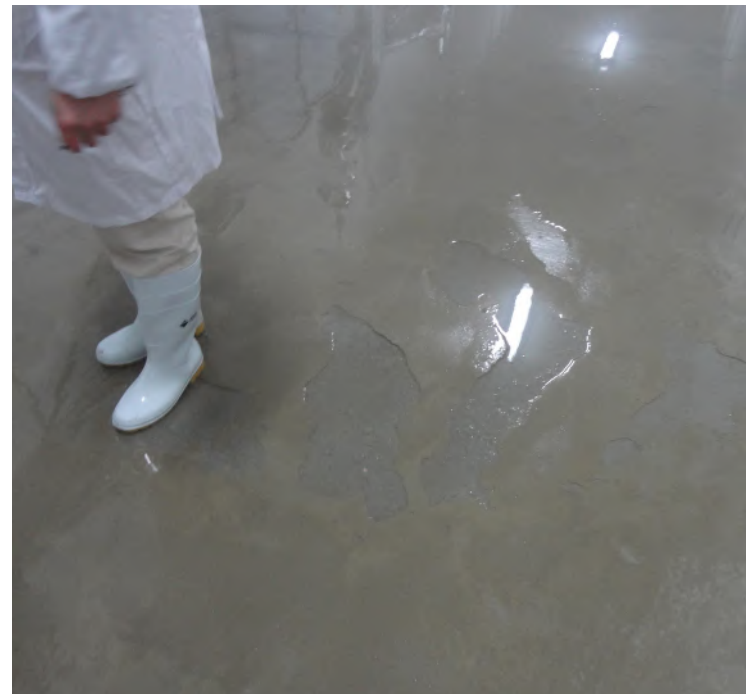
The facility floors should be designed to drain well, prevent standing water and free of cracks and holes. Here, cracks and chips in the floor hold water and prevent the floor from completely drying.
