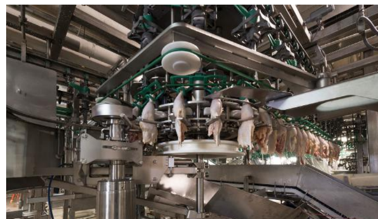
Automated lines maximize labor, have higher volumes of product, less handling (contamination) and maximize floor space.
