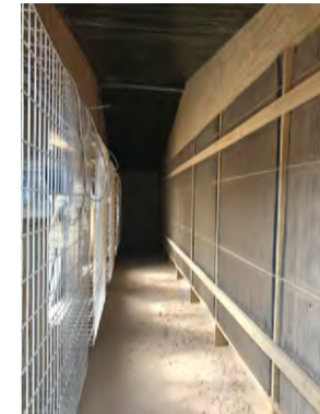
Light trap in a false wall in front of tunnel fans.
