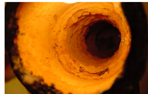
Biofilms and organic material can build up in water lines over time leading to reduced water flow.
